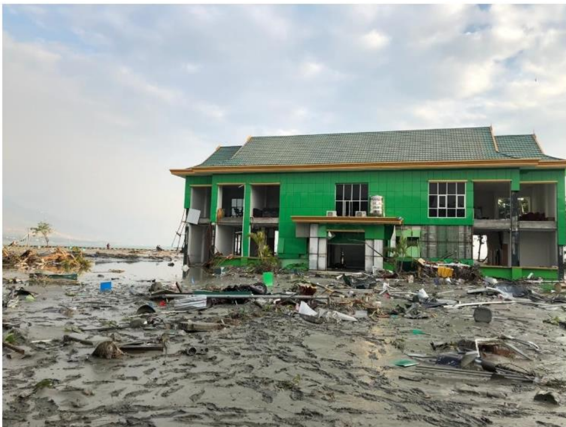
A still-standing building is surrounded by the rubble of houses flattened by the 7.4 strong earthquakes in Palu on Friday. Courtesy of the BNPB (Bnpb/Bnpb)
