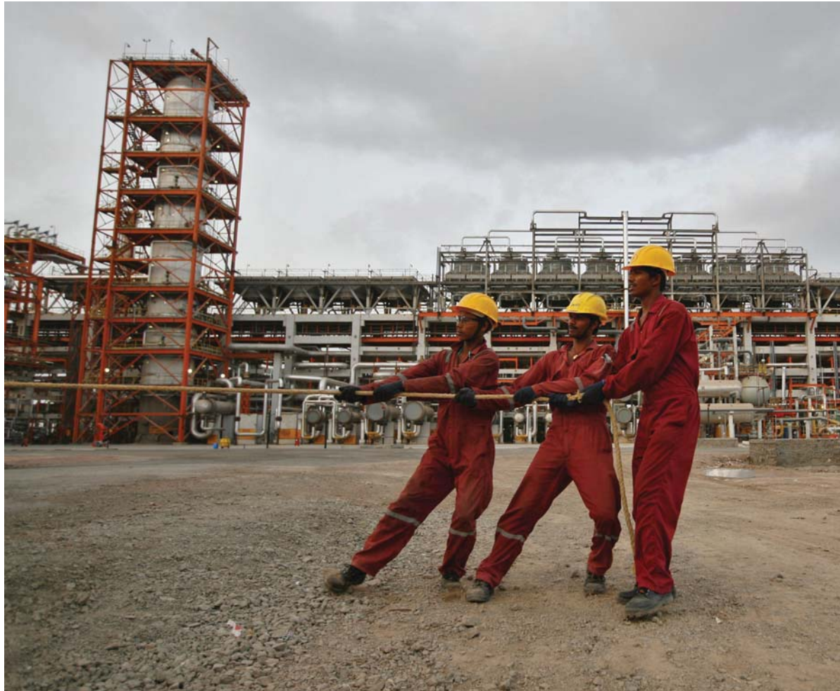
Workers pull a rope to shift an insulated pipe inside the complex of the Vadinar refinery, operated by Essar Oil Ltd (EOL) in the western Indian state of Gujarat.
