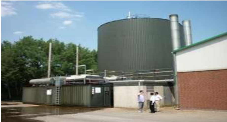
Biogas plant generating 1 MW of electricity and 1 MW of heat plus organic fertilizer
