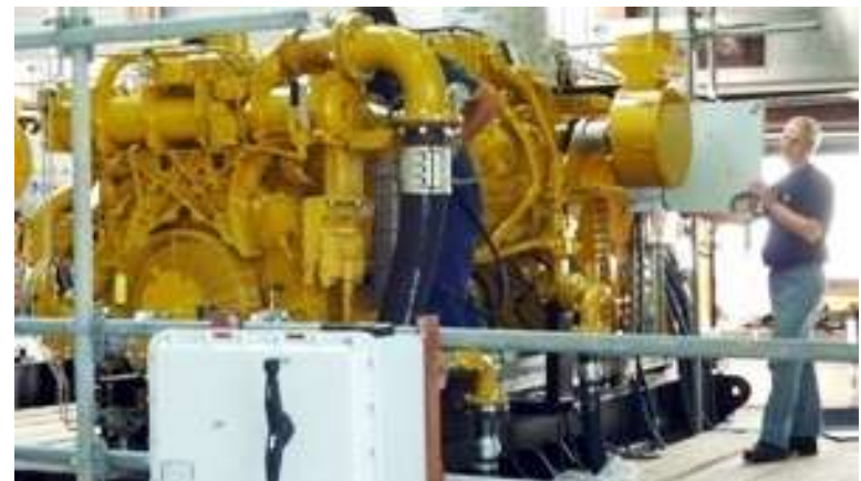
1.5 MW biogas engine generator set
