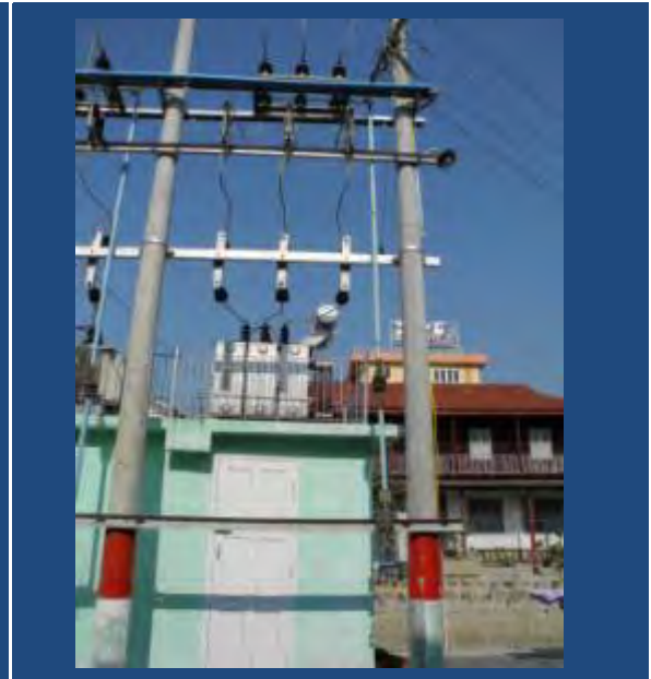
Well maintained installation of the Committee's distribution system
