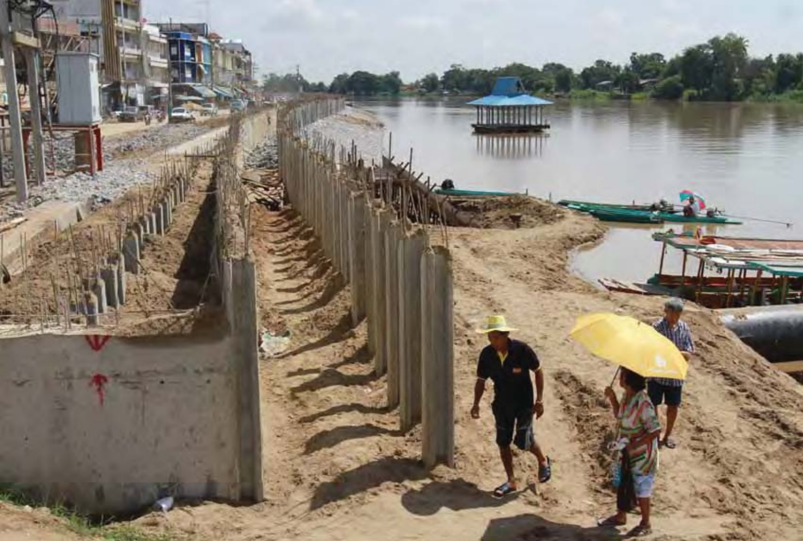
Concrete dikes serve as a flood wall along the Chao Phraya River in Nakhon Sawan, Thailand: Resilience to disasters is an important aspect of national water security.
