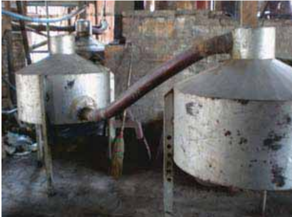
Figure 33: Small-Scale Rice Husk Gasifier in a “Pwat Yay” Factory, Tagaung
