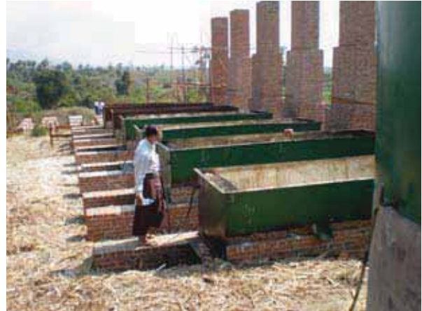
Figure 32: Cane Juice Boiling Tanks of the Ethanol Plant Under Construction in Tagaund Township
