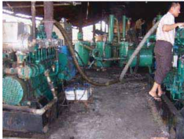
Figure 36: Wood Chip Gasifiers and Generators at JLC, Mandalay
