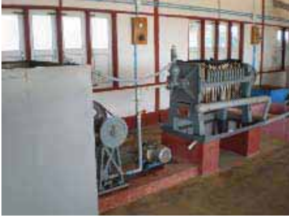
Figure 25: Newly Built Batch Type Jatropha Oil Processing Plant in Man Pan Project (Hill 5), Lashio, Shan State
