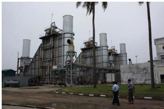
Ahlone Combined-Cycle Gas Turbine
