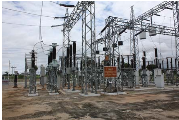
132 kV Switchyard at Magwe
