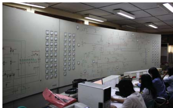
Load Dispatch Center
