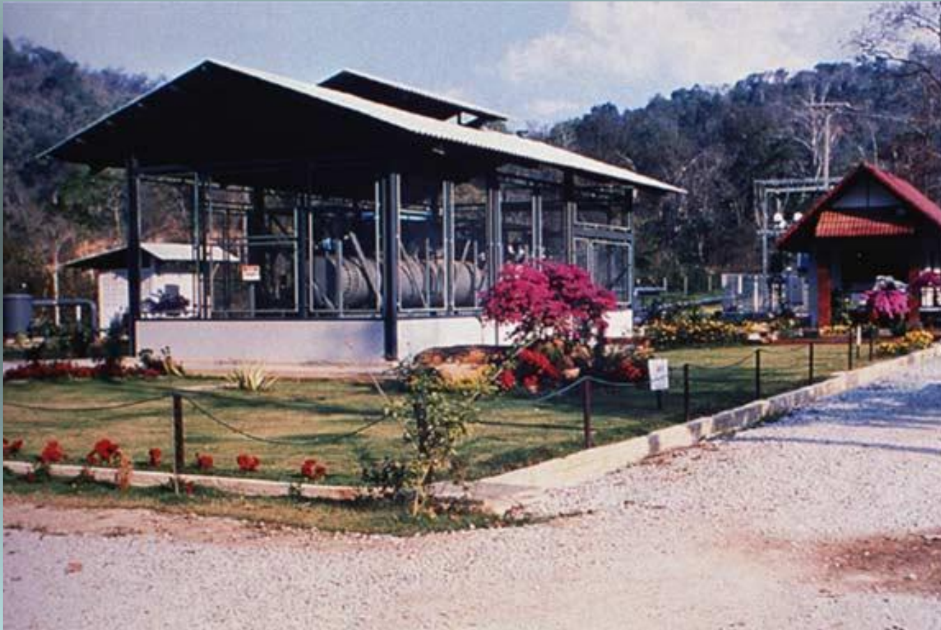
This small binary power plant is in Fang, Thailand.
