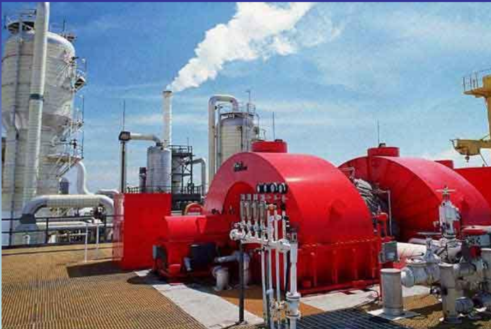
Turbine generator outdoors at an Imperial Valley geothermal power plant in California.
